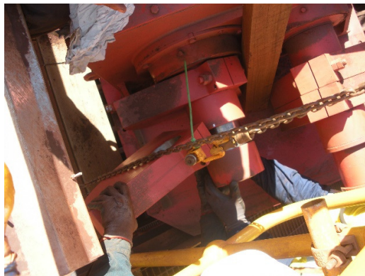
Photo No 23: Spacer piece removed from shaft
